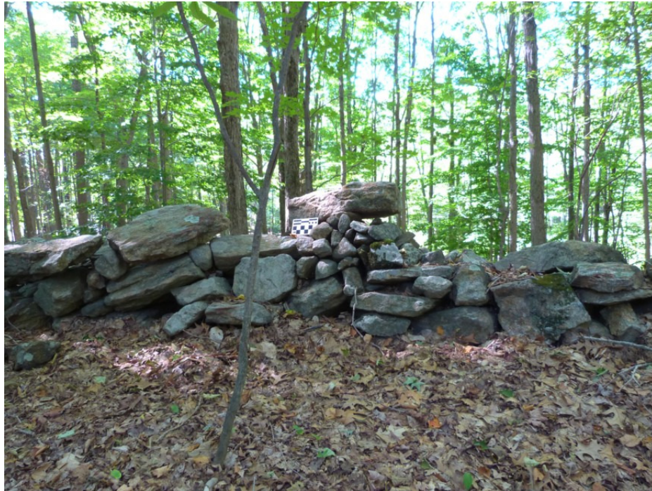
Fig. 33 – The feature is out character with the rest of the wall’s construction (looking to the west)
