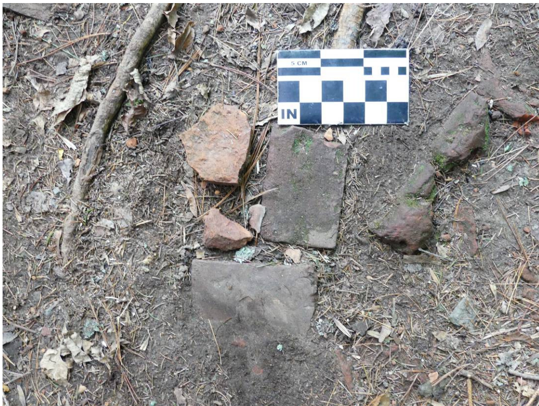
Figure 56 – Broken bricks and coal ash were used to fill the breached section of the tow path/berm.
