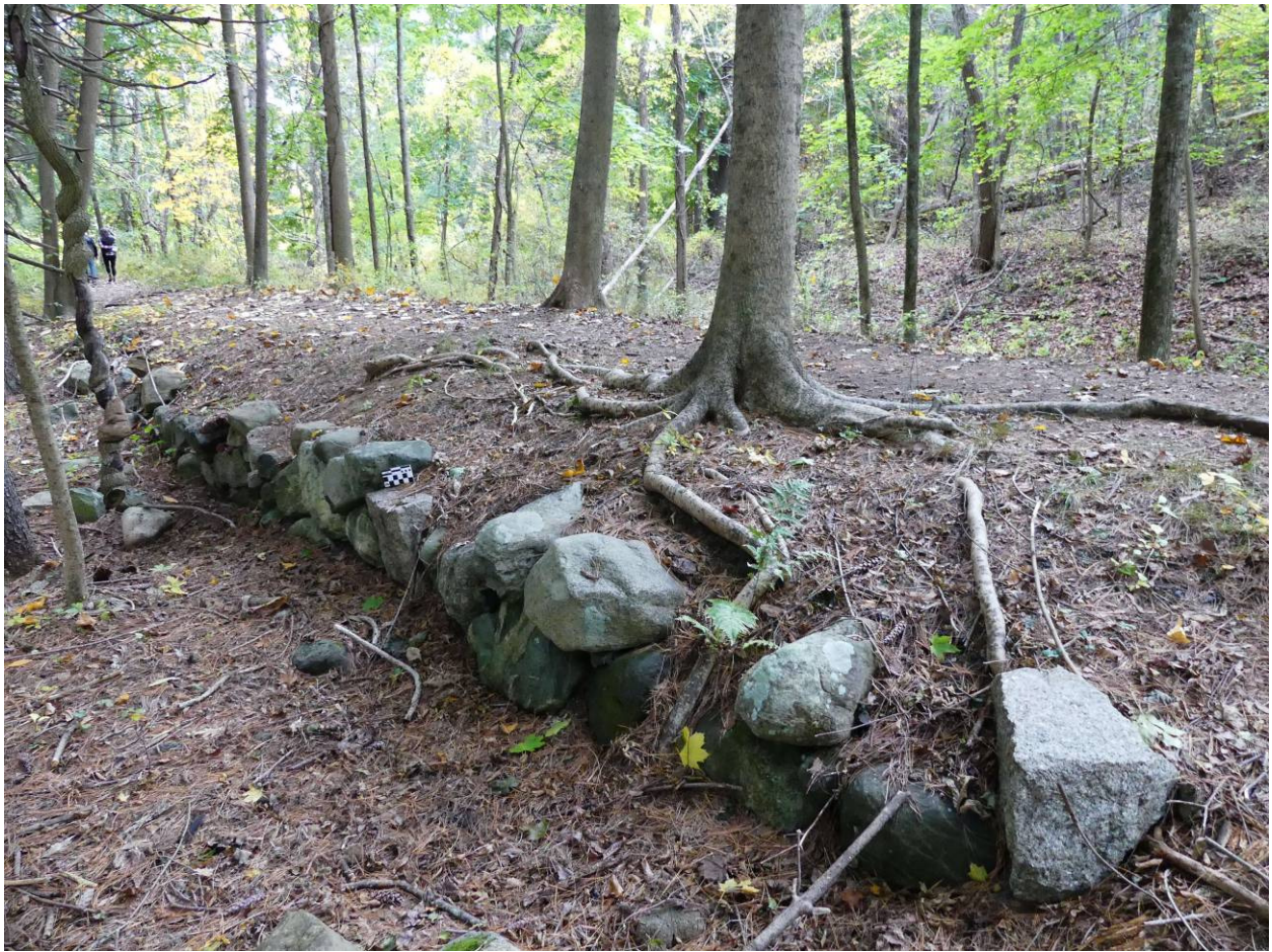
Figure 57 – The retaining wall along the outside of the tow path/berm where it had been breached.
