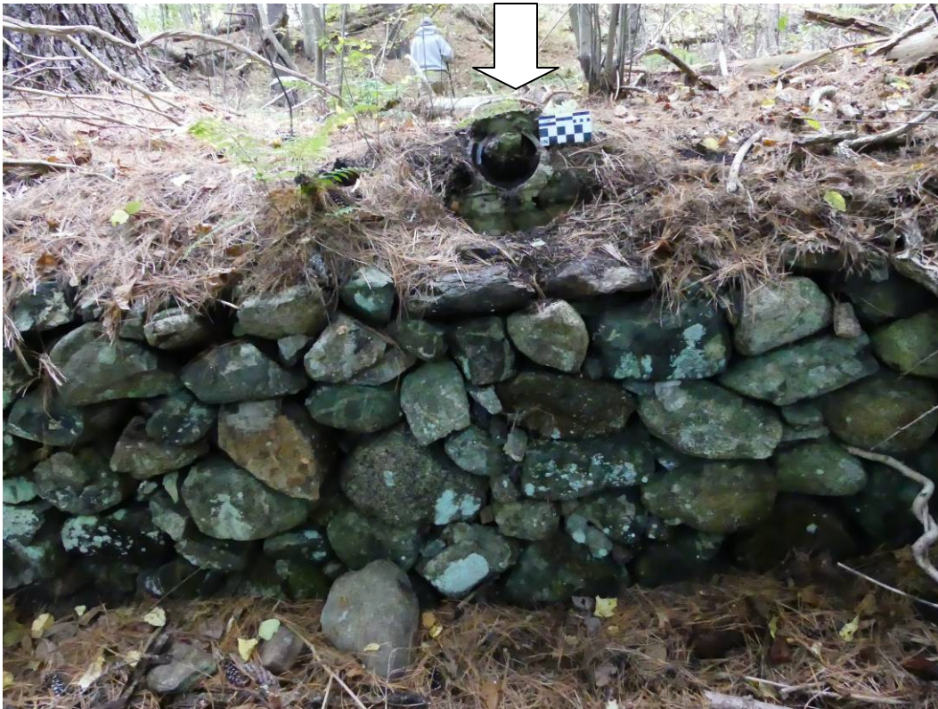
Figure 61 – West wall of house cellar. It is dry masonry construction. Arrow indicates terracotta pipe entering the house.
