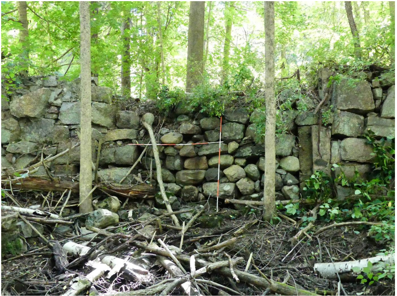
Figure 3 – Intake opening into mill foundation now filled with stones.
