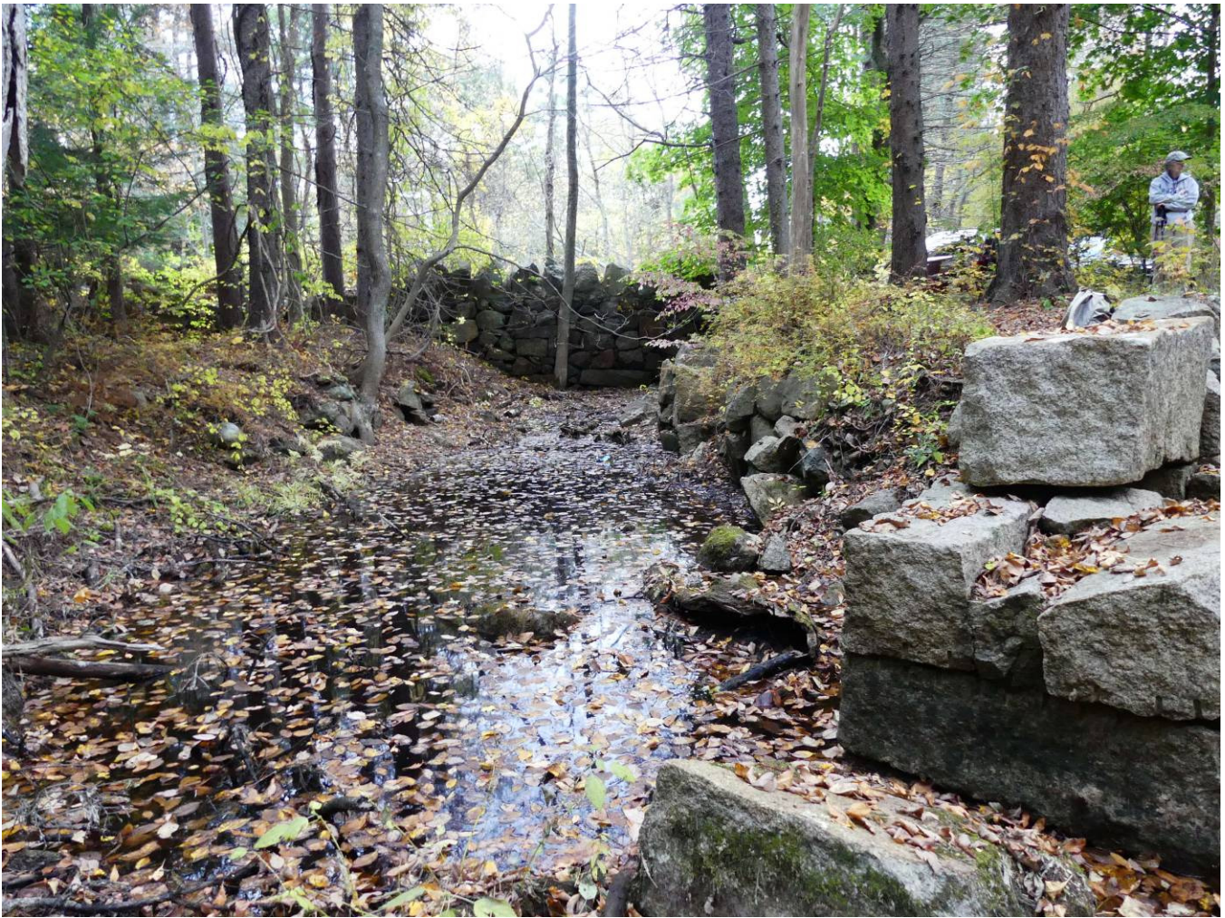
Figure 24 – Tailrace: View from the mill foundation (culvert on right side of photo) looking northeasterly towards Winthrop Street.
