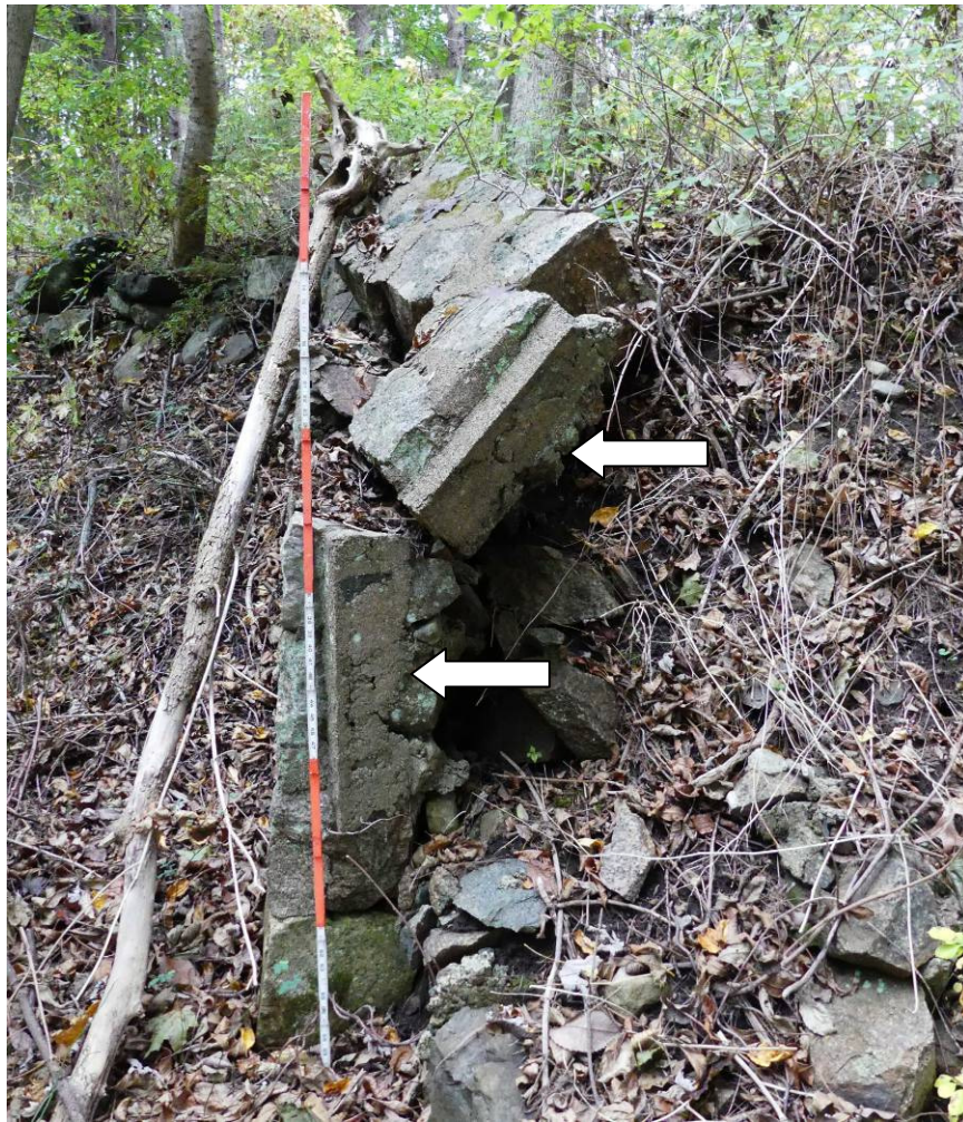
Figure 31 – View of end of angled stone and cement wall showing form poured cement feature.
