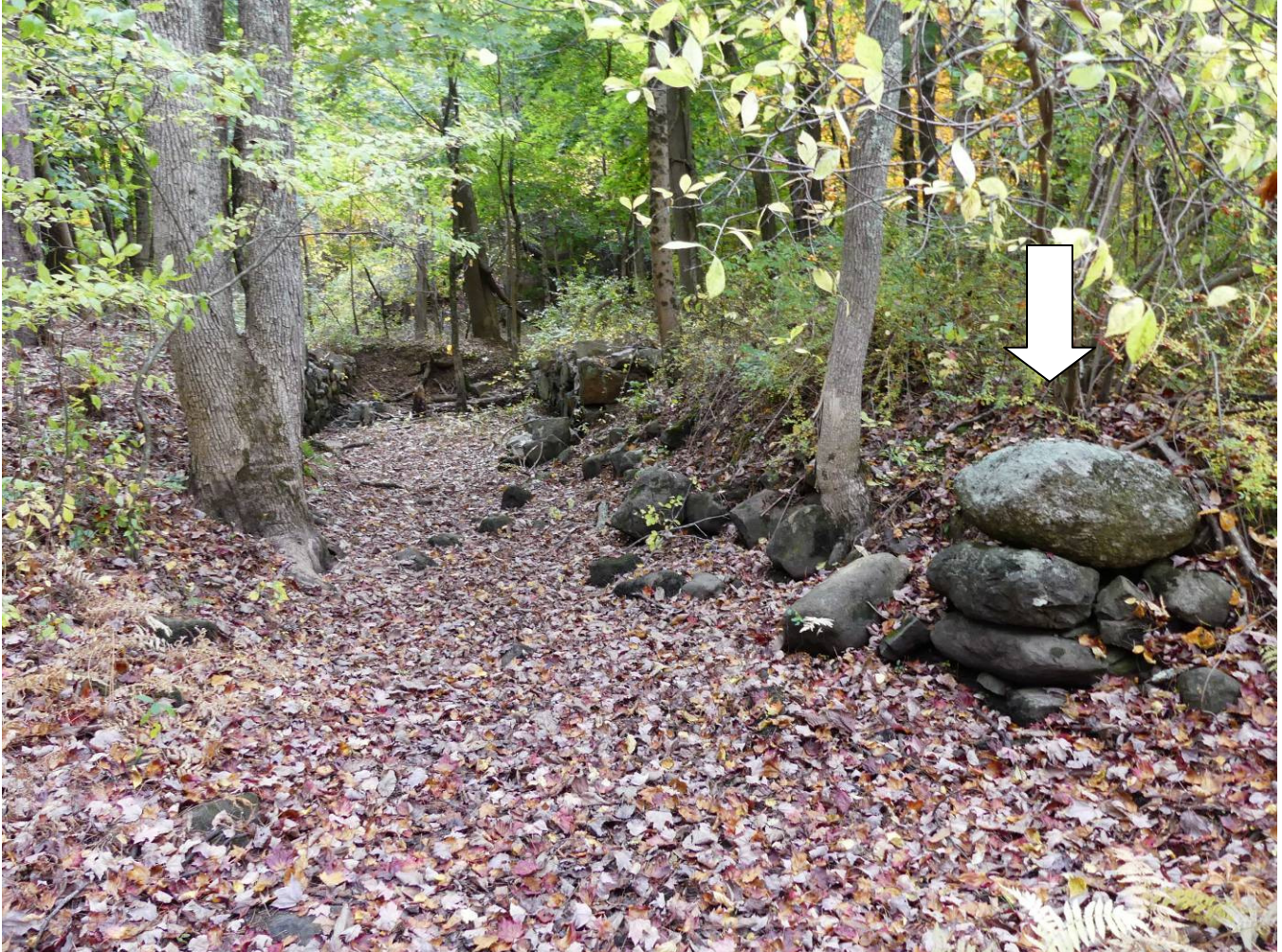
Figure 45 – View of tailrace from bank of the Ipswich River. Many of the stones in the tail race retaining wall have fallen down. The end of the tailrace wall on the right finished with large field boulders (arrow).
