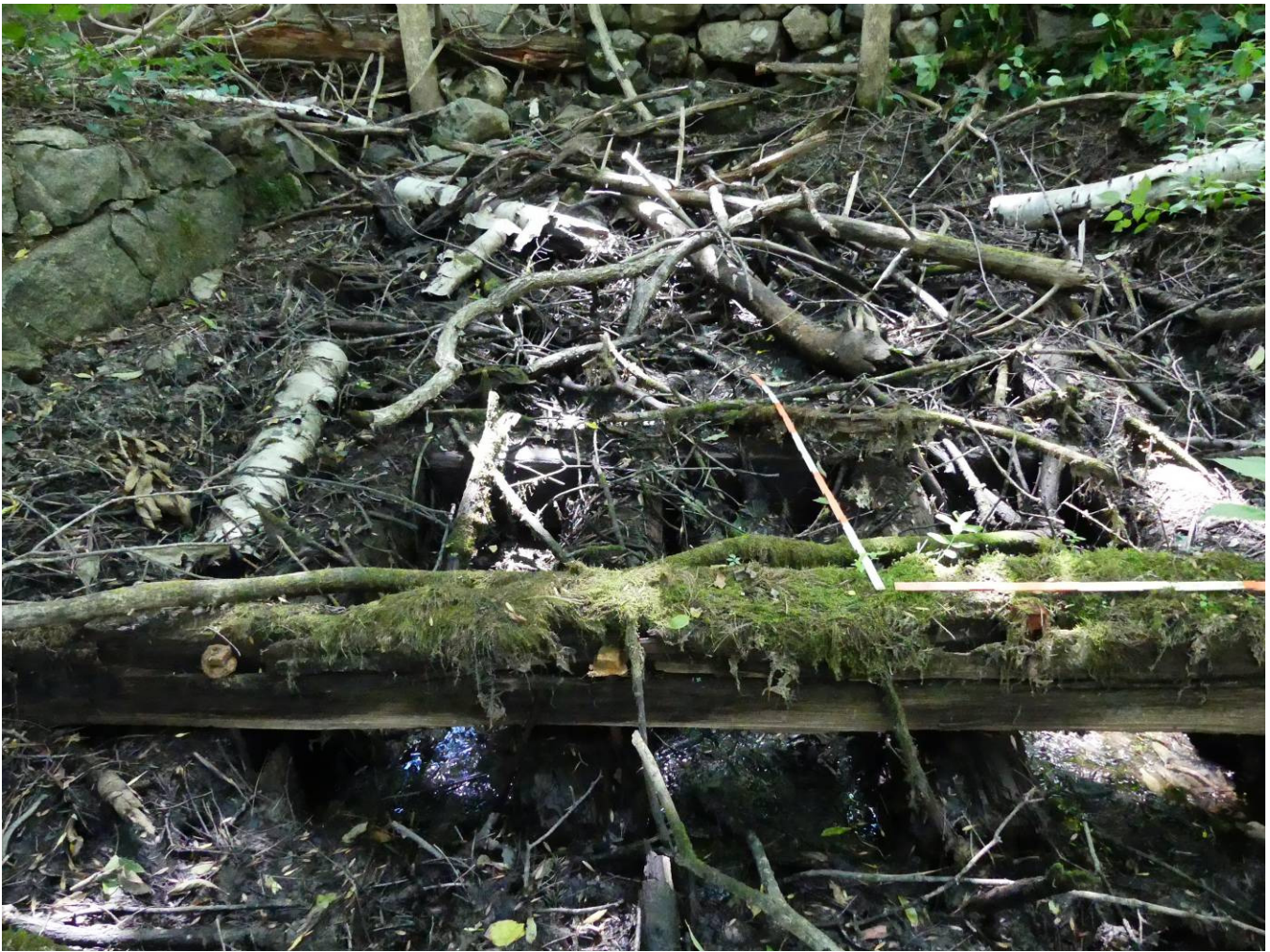
Figure 8 – Across the lower bottom of photo is a large timber part of a grid of timbers that support the turbine. The timber grid is located on the ground north of the water intake opening and next to the 1 st low stone wall.
