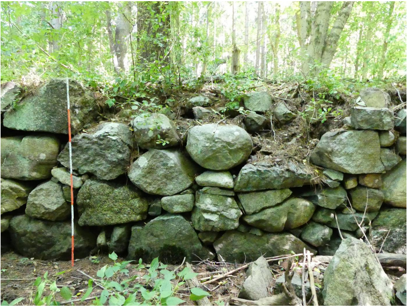
Figure 42 – A collapsed section of the foundation wall shows its backfilled stone rubble.
