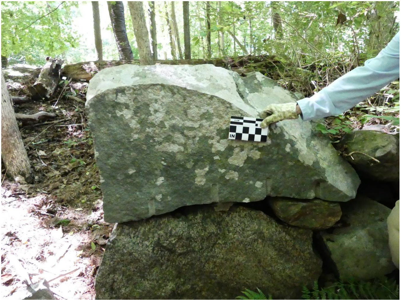
Figure 40 – The flat sides of the split field stones were arranged to create a flat face to the foundation wall.
