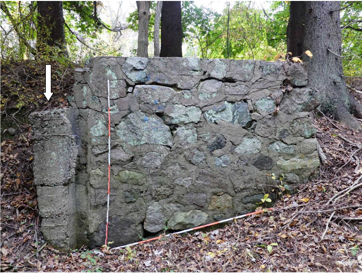
Figure 28 – Stone and cement retaining wall at end of canal. Arrow points to form poured cement feature. (View from inside canal)
