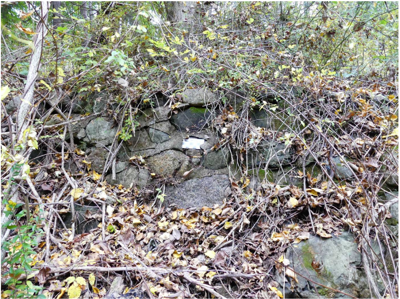
Figure 33 - Stone and cement retaining wall along top edge of earthen berm / tow path.
