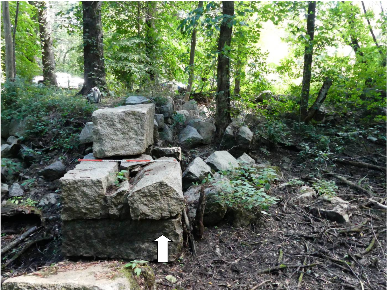
Figure 14 – Side view of culvert. Note the oddly shaped block of stone (arrow). This is considered “waste” or “grout” at commercial stone quarries.
